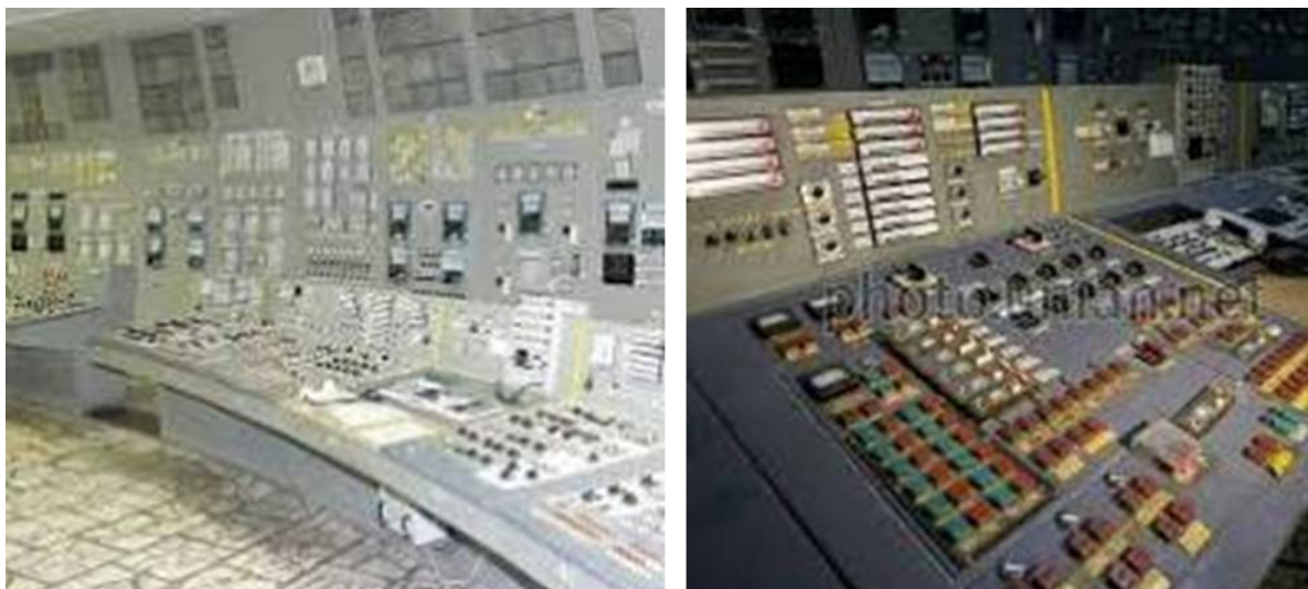
Figure 2. Control panel of the 3-rd and 4-th power units of the Chernobyl NPP
